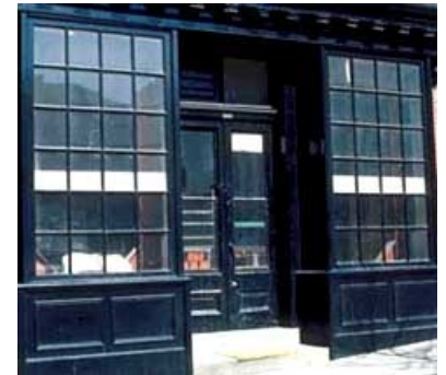
This cast iron storefront from the late 19th century has been well maintained over the years. Photo: NPS files.
