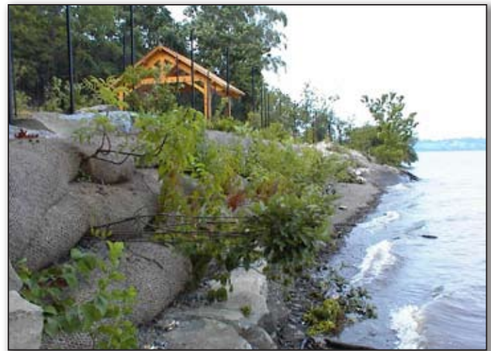
Installed vegetated shoreline stabilization treatment with native plant species, biodegradable soil bags, and a sloped shoreline.
