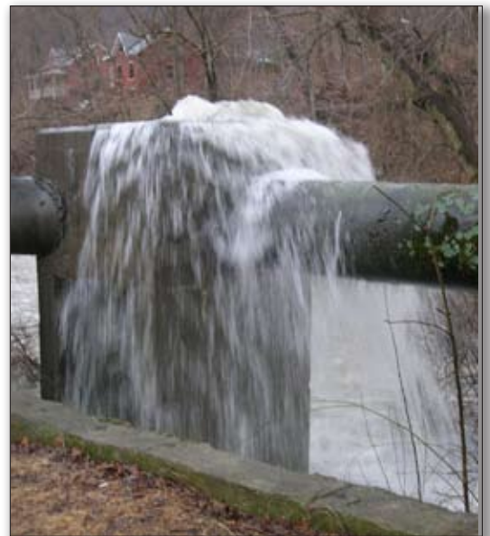
Aged infrastructure that is beyond capacity.
