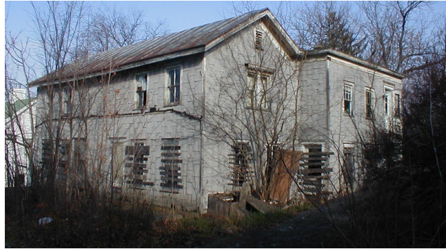
Figure 6: Mill District House in Need of Repair
