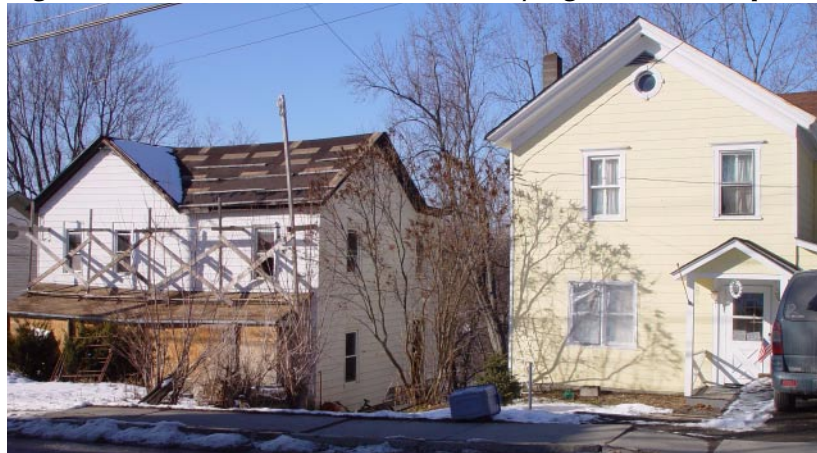
Figure 12: Main Street Houses in Varying States of Repair
