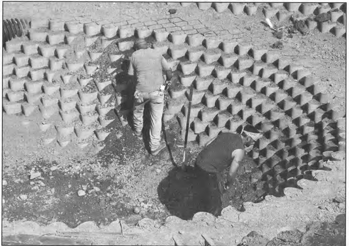
Workers put the finishing touches on the drainage project in Wappingers Falls.
