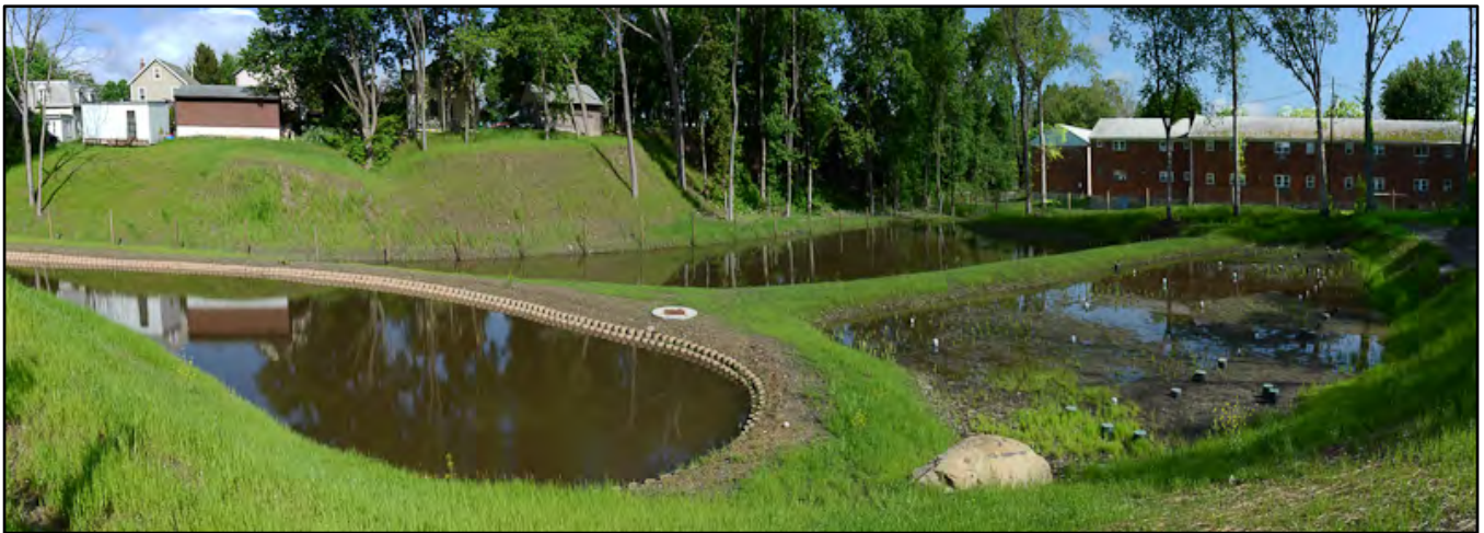
After heavy spring rains, retention pond full, outlet overflow pond full, April 2014
