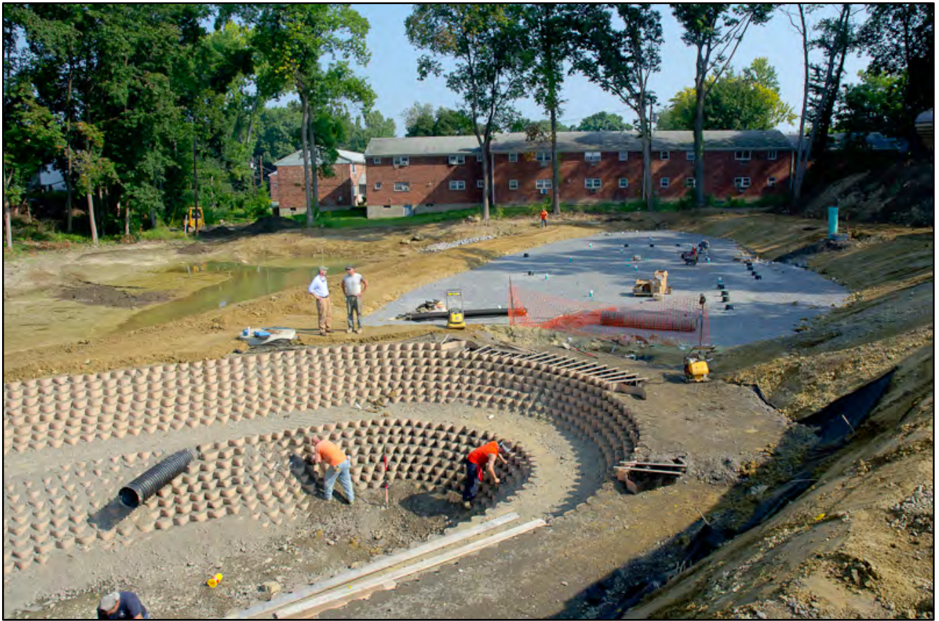
Sedimentary forebay (retention pond) in foreground, with gravel wetland filter above and outlet pool on right
