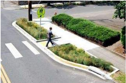
Permeable pavement, bioswales, planter boxes, and trees are among the elements that can be woven into street or alley design.
