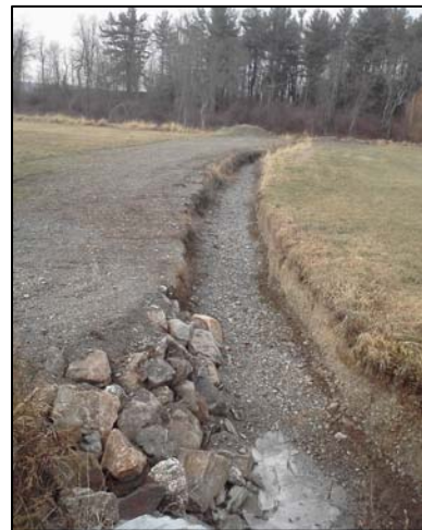
Unprotected drainage ditch
