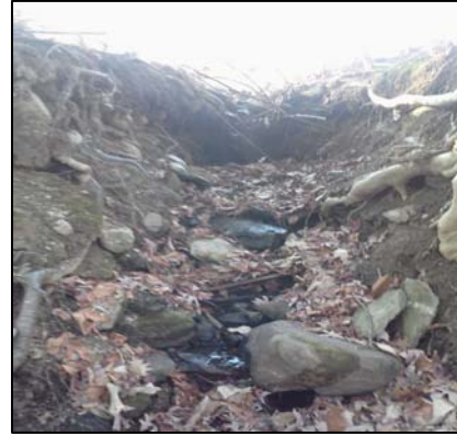
Taconic State Parkway Eroding Ditch
