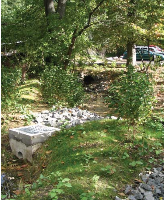
Stormwater treatment, Westchester
