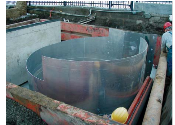
Stormwater treatment system
