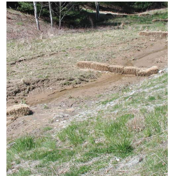
Improper use of control measures
