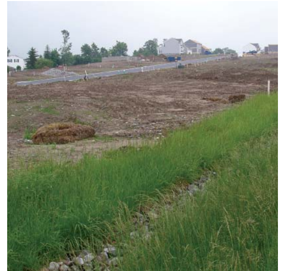
Construction site erosion
