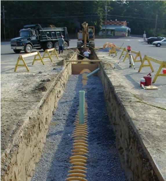
Stormwater treatment installation
